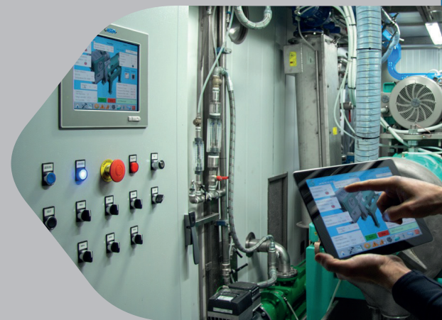
Remote Monitor and Control System
